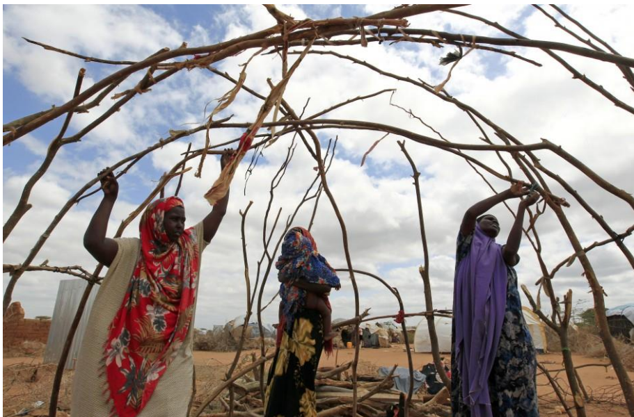
Figure 10. Image of a refugee built shelter 1. (International Business Times, 2011) The photo to the right shows women building a makeshift shelter, while the photo below shows the end product.
